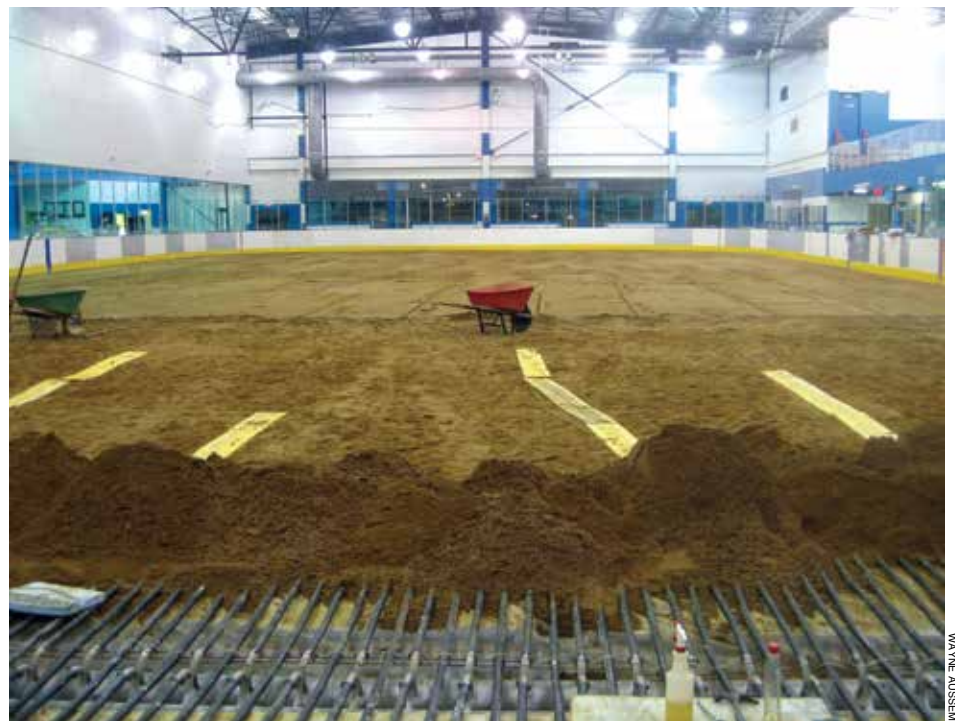
Secondary refrigeration cooling piping, as seen prior to leveling.
